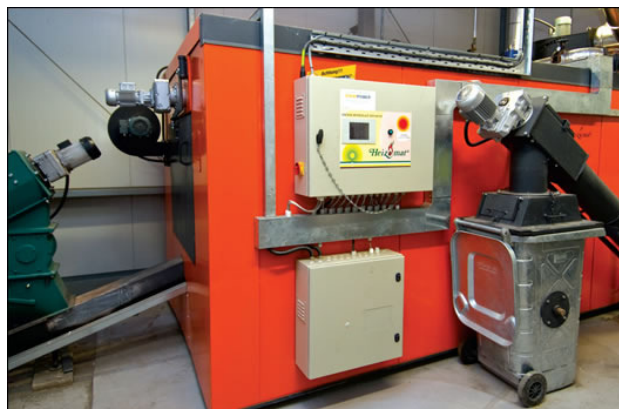
Heizomat RHK AK 650 boiler at IKEA
