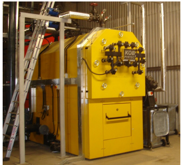
Viessmann (KOB) Pyrtec 950kW boiler
